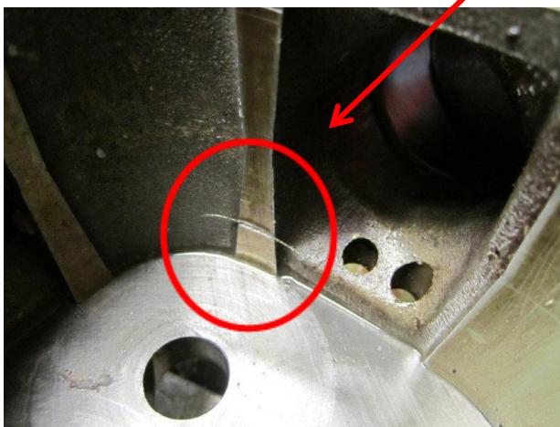
Wire from strainer that caused meter lockup
