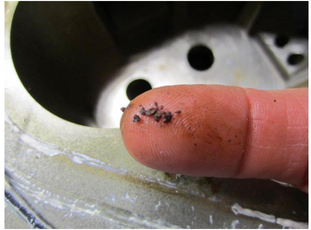
Rust particles that caused meter lockup
